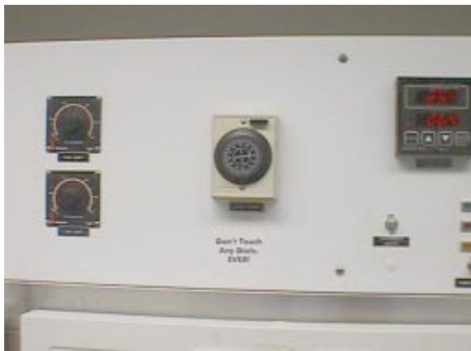
Figure 1. The control panel for the large double-door incubators in the Mueller and Rose labs.
